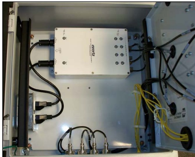
Figure 2-7: 2400ODU Fiber Cable Routing
